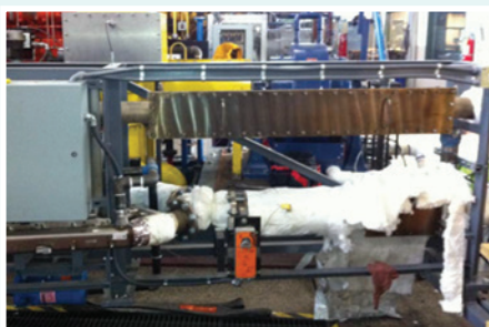
Catalyst Slipstream System
