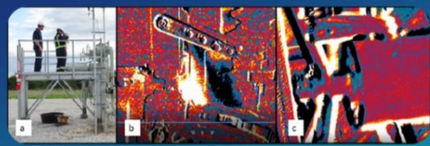
As part of PR-746-22204-R01 Review of Technologies to Enable In-situ Valve Service to Reduce Methane Emissions (a) WVU researchers surveying components for leaks, (b) example of leaking packing on automated control valve, (c) example of leaking packing on manual isolation valve.
